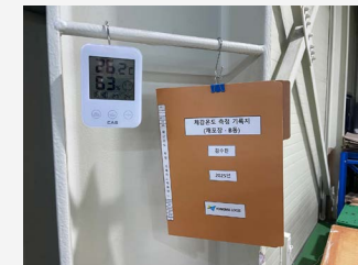
Installation of Temperature and Humidity Monitors
